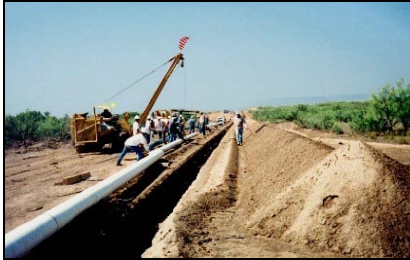
Figure 4-6: Val Verde Pipeline, Petro Source Carbon Company, cited October 11, 2002 at http://www.petrosourcecorp.com/HP_co2/
