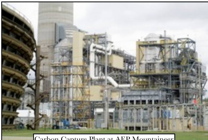
Carbon Capture Plant at AEP Mountaineer
